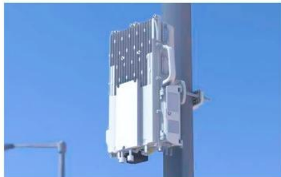
5G base station
